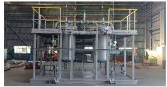
Filter Skid (LGC GTC)
