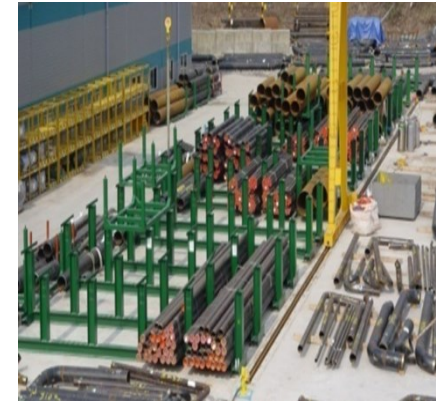
3. Storage / Material Handling
